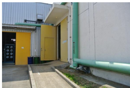
Steam pipes running inside the premises at Nikon Imaging (China) Co., Ltd
