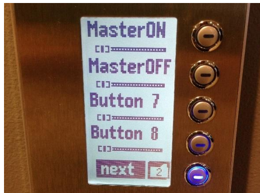
Main control panel for lighting at Nikon Australia Pty Ltd
