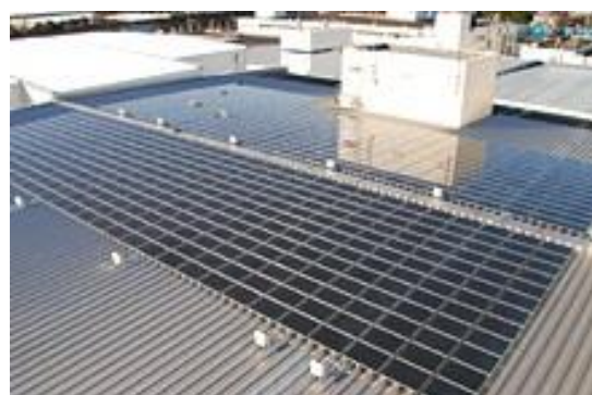
Solar power generation panel at Kumagaya Plant
