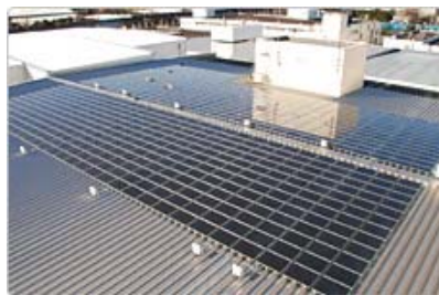
Solar power generation panel
