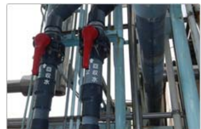
Pipes through which the recovered and treated water is supplied to the washing process (at the Sagami-hara Plant)
