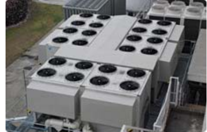
Heat pump chiller equipment of the seamless HVAC system
