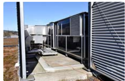
Heat pump system at Nikon AG
