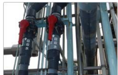
Pipes through which the recovered and treated water is supplied to the washing process (at the Sagami-hara Plant)
