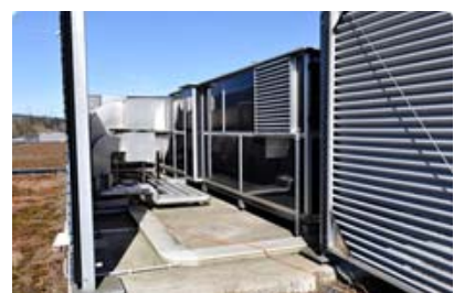
Heat pump system at Nikon AG
