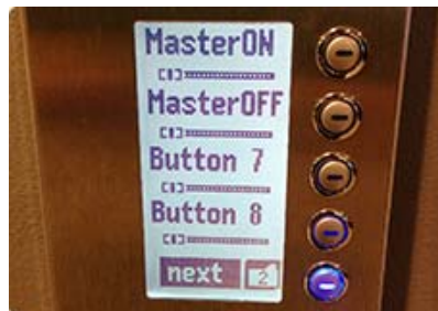
Main control panel for lighting at Nikon Australia Pty Ltd
