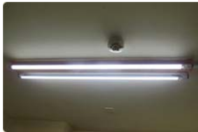
Nikon Imaging (China) Co., Ltd. Fluorescent-style LED lighting in common areas
