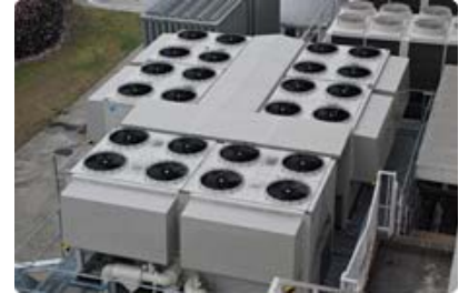
Heat pump chiller equipment of the steamless HVAC system
