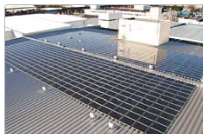
Solar power generation panel
